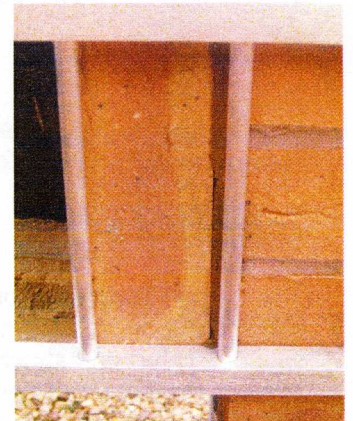
Each brick is laid behind Laurens Ladder using the top bar as a level and the vertical bar as a mortar joint gauge
